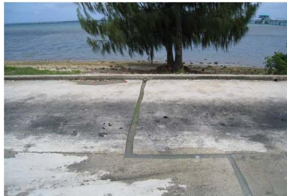
Figure D-12. Runoff from the concrete bus loop is conveyed across the concrete pad via grooves and sheetflow, and discharges through square notches in the curb to the nearby beach and water. There are oil stains on the concrete pad and bus exhaust deposits other pollutants on the concrete.
