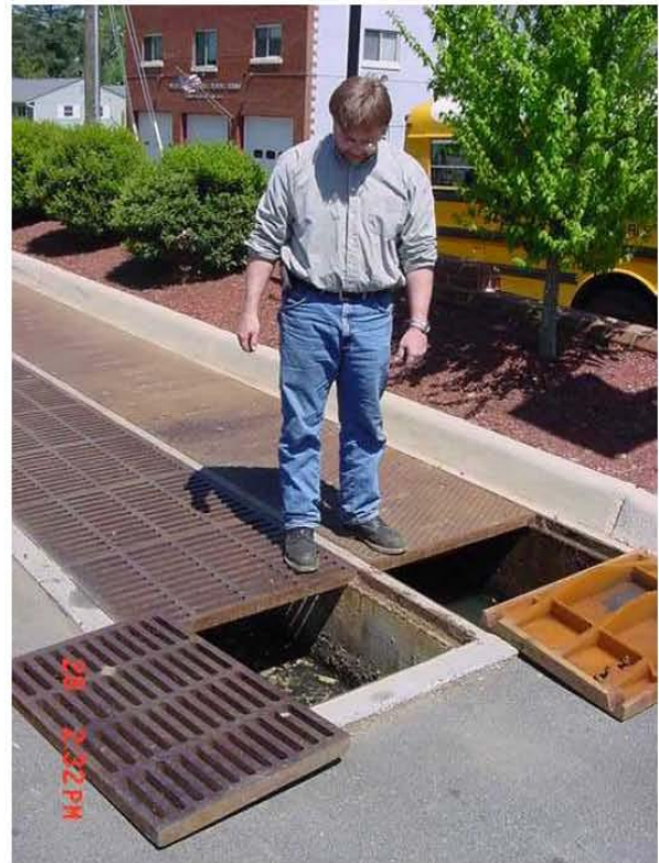
Figure D-15. Example of sand filter with grate top. The grates provide maintenance access.
