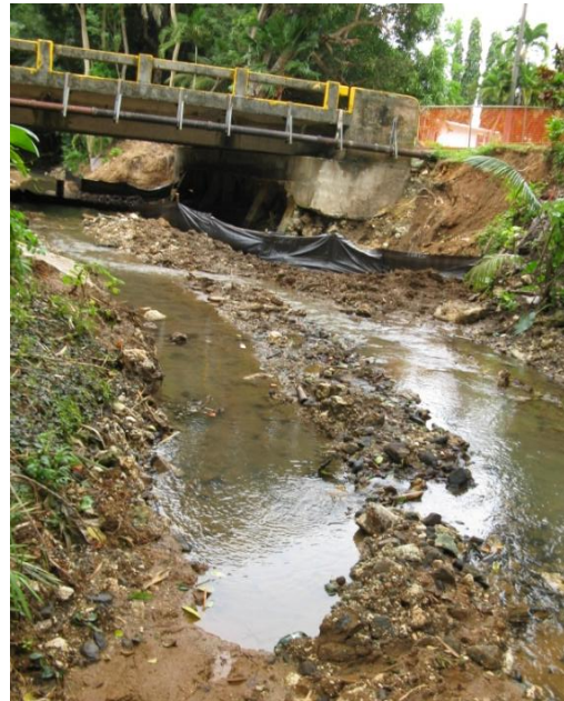
Figure 37. Example of a poor construction practice at the Masso bridge. A backhoe drove into the river bed destroying the river bed structure. Sediment fences along the bridge were only installed after the contractor was cited. Photo courtesy of David Burdick.
