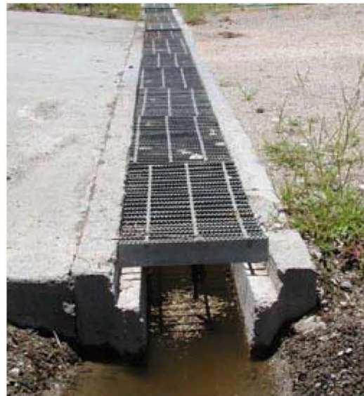
Figure D-24. Example of a trench drain that can be used to convey runoff from parking area to bioswale.
