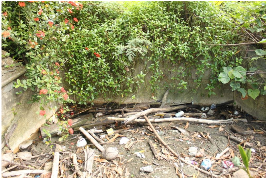
Figure 39. Clogged culvert along Marine Corps Drive in Piti.
