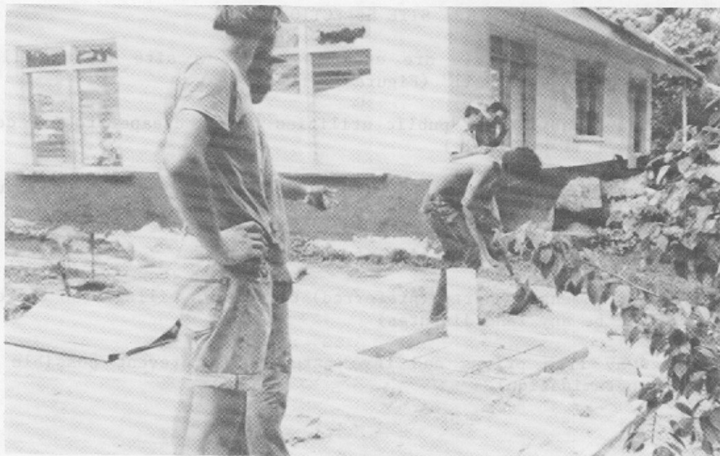
Figure 8. Pouring a slab to seal an existing well for a modified "WERI WELL" installation.
