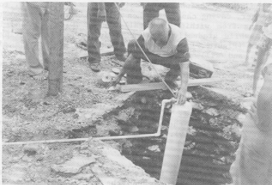
Figure 7. Use of an existing well for a modified "WERI WELL" installation.
