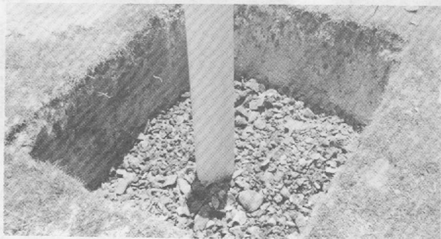
Figure 17. Backfilling with aggregate, step 2. Carefully place aggregate in the well around the 6-inch pipe until it reaches the water level.
