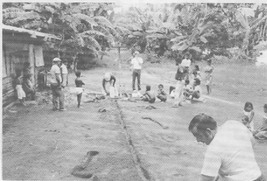
Figure 36. Running the \frac{1}{2} -inch PVC pipe. Run pipe from the well to the tank location. The pipe should be buried slightly below the ground to help protect it from damage.
