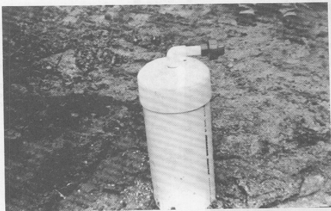
Figure 27. Installing the union/elbow assembly. Use PVC glue to attach the elbow end of the assembly to the well pipe. (Note: before gluing, rough edges of the pipe end should be removed with a knife and the end of the pipe should be sanded lightly). After gluing, the elbow will rest on the well cap keeping the pump 6 inches from the aggregate at the bottom of the well.
