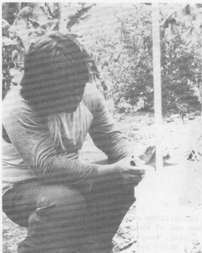
Figure 25. Measuring the well pipe. Lift the well pipe/pump assembly 6 inches off the bottom of the well and mark the pipe where it comes out of the well cap (photo on the left).
