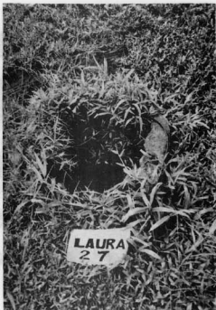
Figure 28. Well made of a drum can, Laura well #27, Majuro. A maintenance problem is illustrated.
