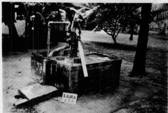
Figure 26. Well made of cement/concrete with a hand pump, Laura well #13A, Majuro.
